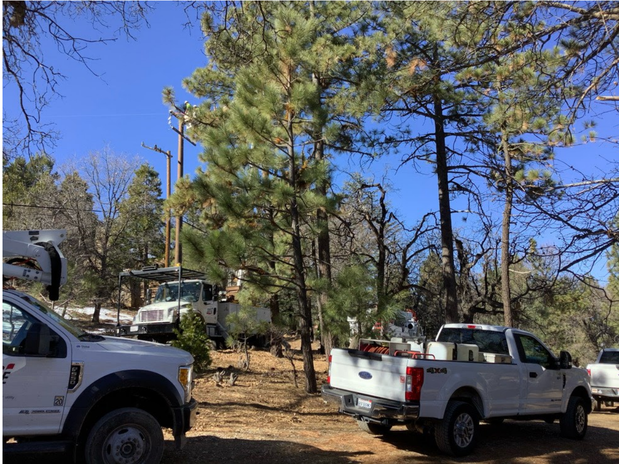
Photo 4: During conductor transfer at Pole P40427 (C 440), a Dedicated Fire Patrol was present and equipped with at least 150 gallons of water with pump and hose in accordance with the CFPPP for conductor work with energized lines on NFS land with a PAL C.
