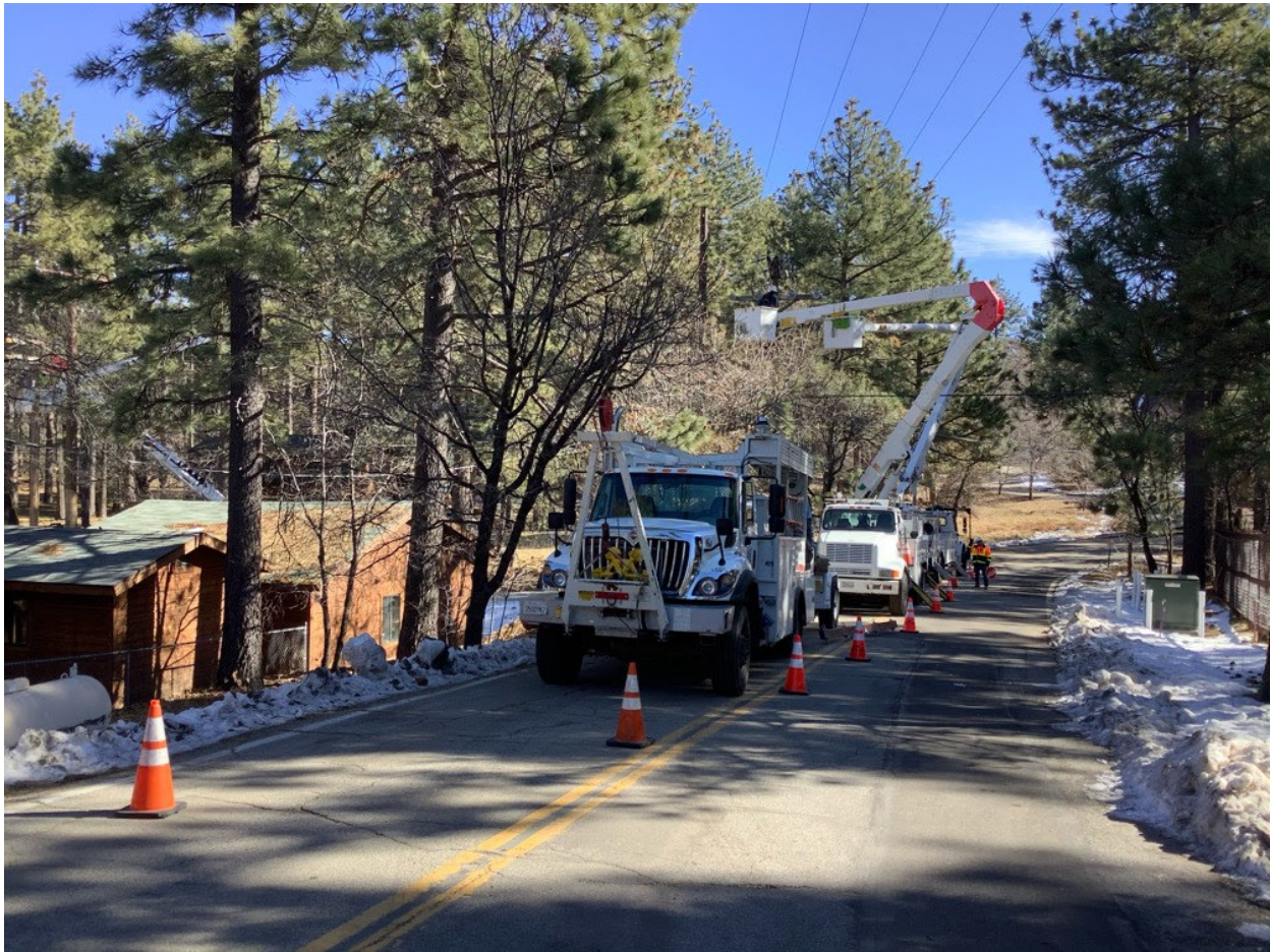
Photo 6: A crew was observed conducting overhead work at Pole P40196 (C 440). Cones, signage, and flagpersons were used to direct one-way traffic safely around the work area in accordance with the TCP and APM TRANS-02.
