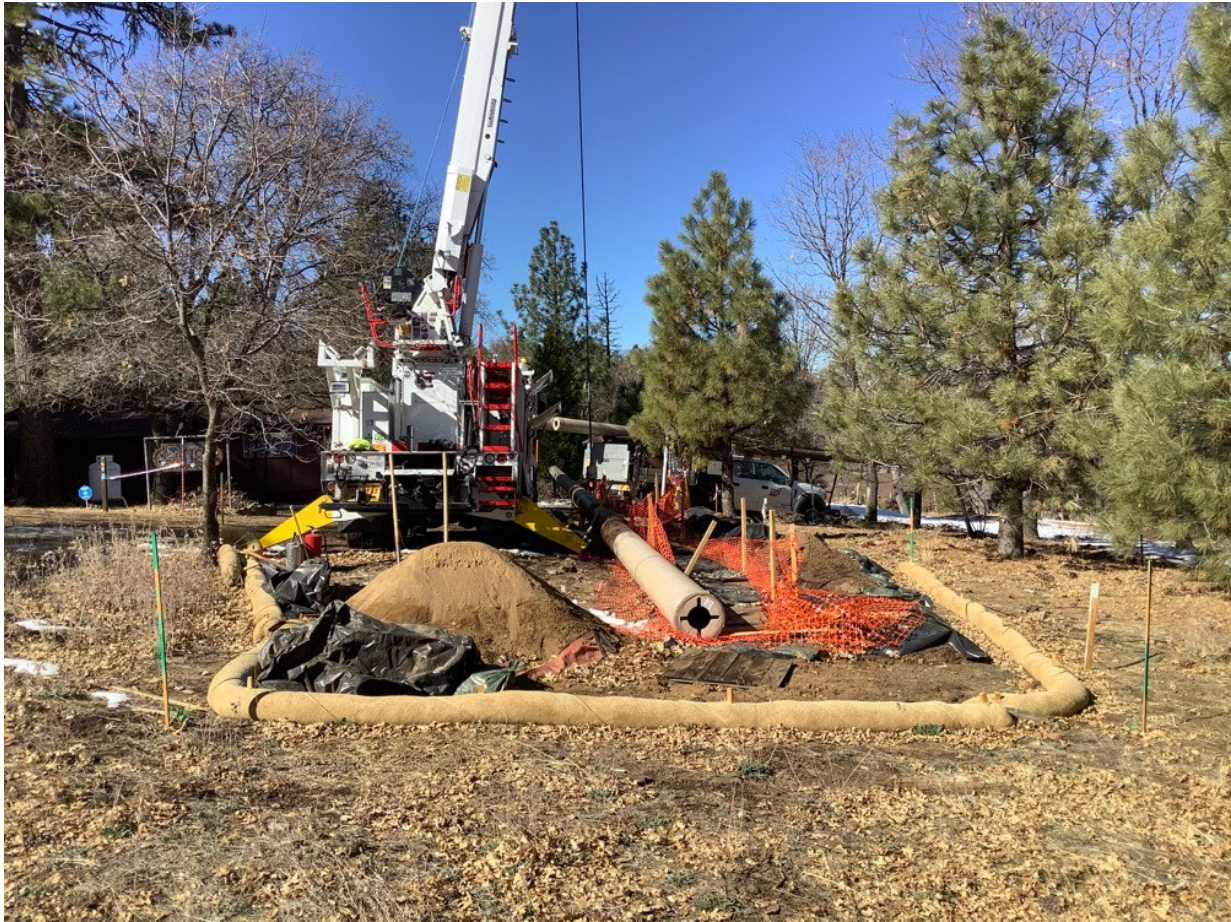
Photo 5: A crew was observed framing and preparing to set Pole P260350 (C 440). Erosion control BMPs at the site were observed in good condition in accordance with the ECP, SWPPP (MM HYD-1 and MM BIO-7), and APM HYD-09.
