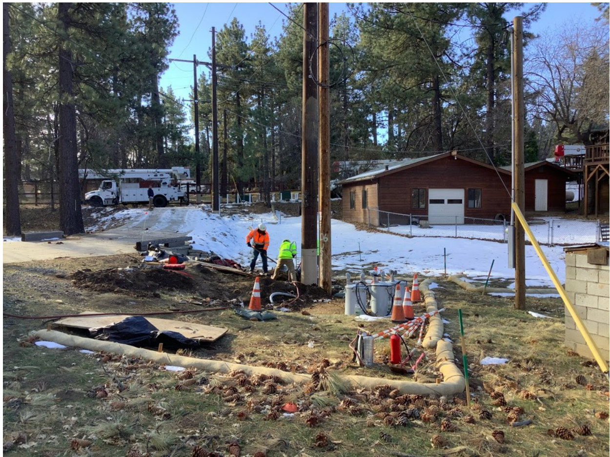
Photo 1: During backfill operations at Pole P40196 (C 440), the crew was observed remaining within clearly delineated work limits in accordance with MM BIO-1.
