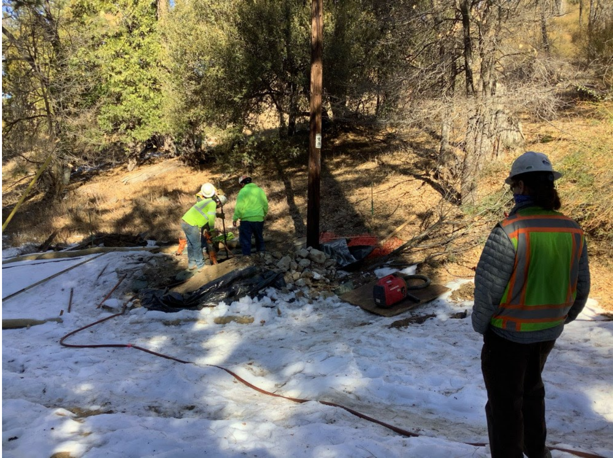
Photo 2: A Biological Monitor was observed monitoring pole hole digging at Pole P40217 (C 440) to ensure compliance with mitigation measures, applicant proposed measures, and permit conditions in accordance with MM BIO-22.
